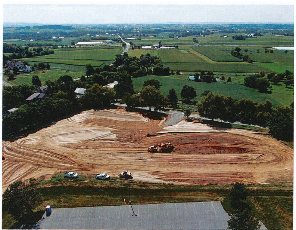
Excavation work last summer began the conversion of a four-acre hay field adjacent to Akron Mennonite Church into a nature preserve. PHOTO: PHIL RUTT
